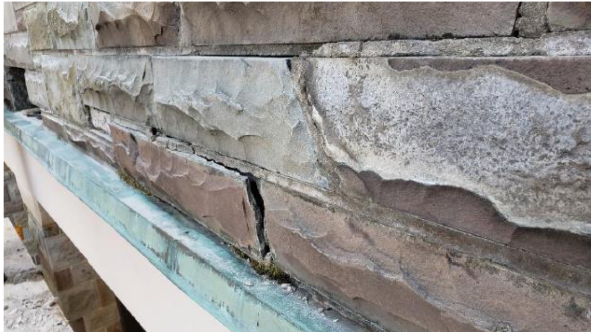
Face of loggia parapet wall showing severely deteriorated condition of veneer, including delamination of (Llenroc) bluestone. MCWB Architects 2020
