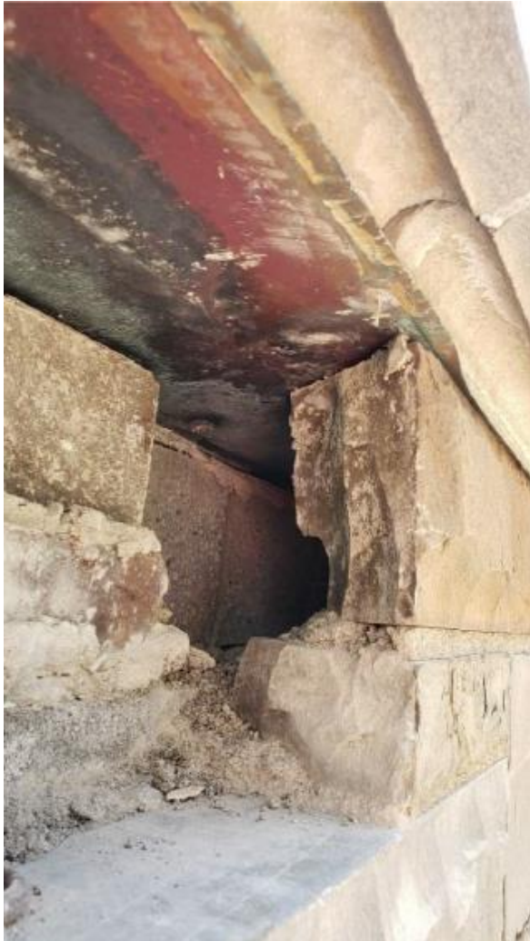
Top of loggia parapet wall. Note cavity and replacement block on roof side, and copper thru wall flashing under coping. MCWB Architects 2020
