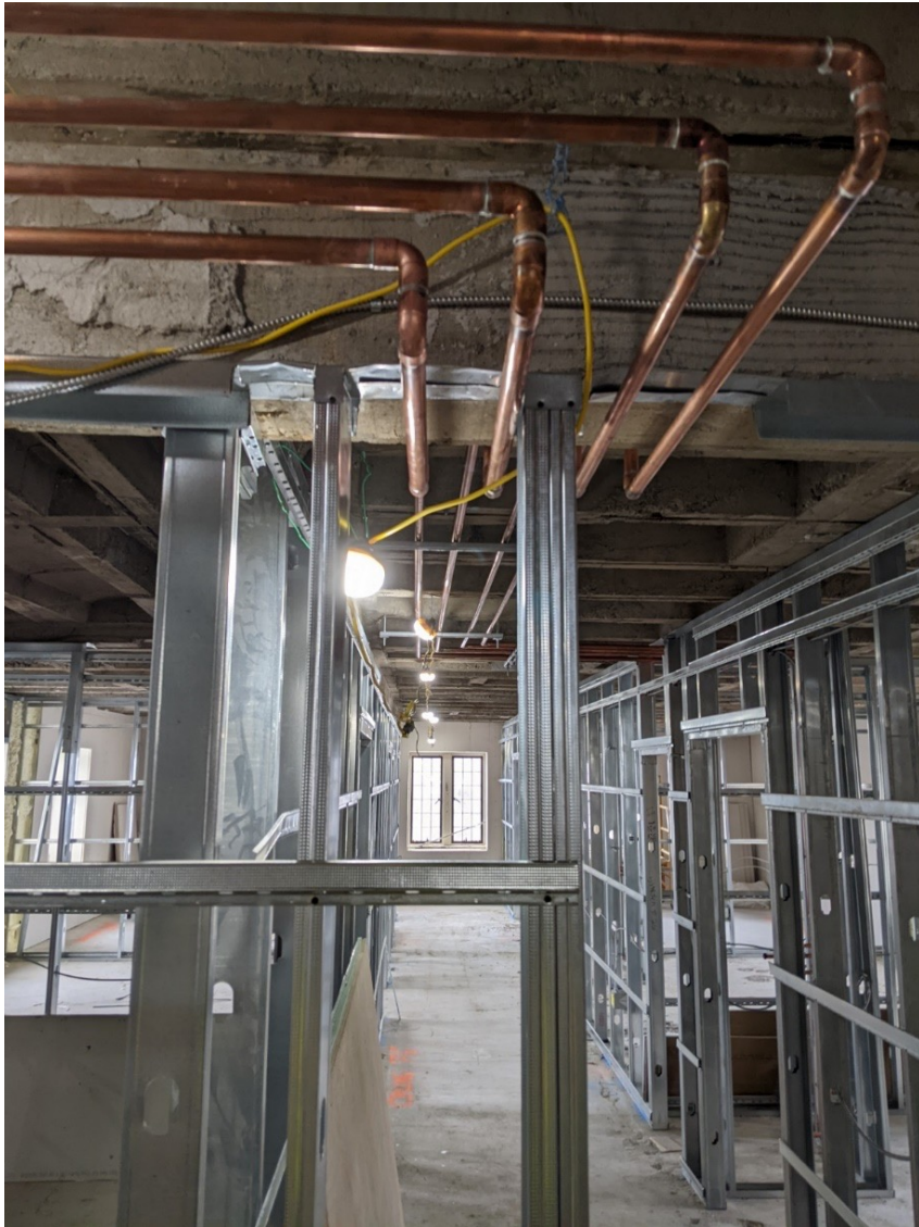
Corridor Room Piping and Framing
